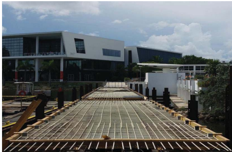
Figure 1.1: GFRP bars in the deck of the Fate Bridge at the University of Miami's campus
